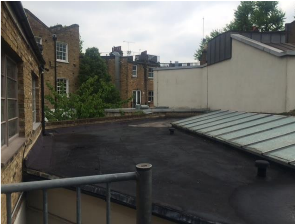
Image 4: View looking east of flat roof over existing single storey element of the building
